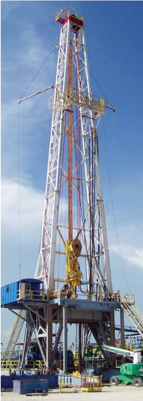
The approximately 150-foot-tall cavern rig is drilling a well deep into the Spindletop salt dome.
